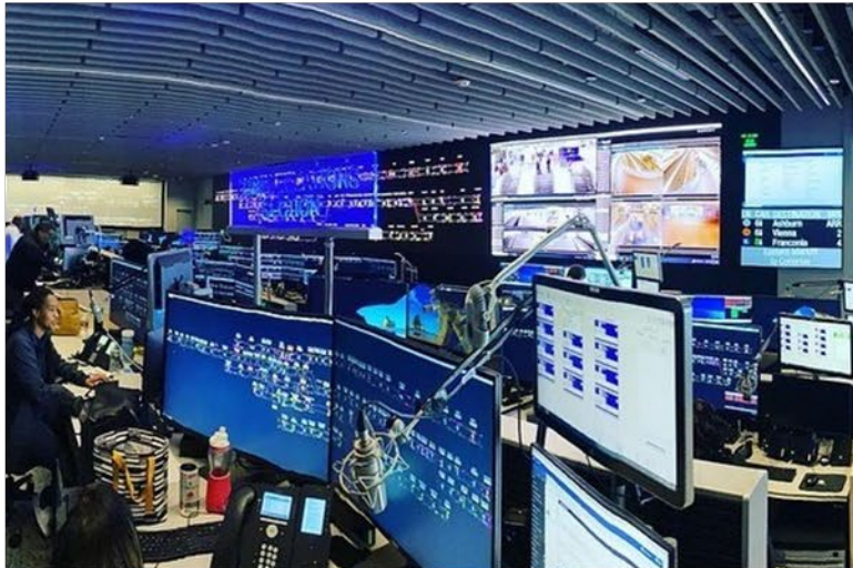
Metro Integrated Command & Communications Center (MICC)
