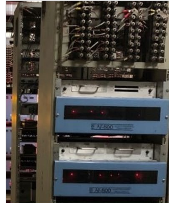
Track Circuit Module
