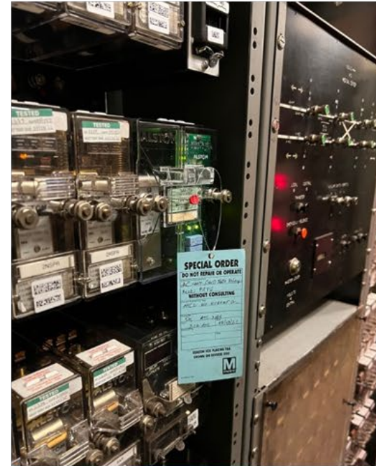
Vital Relays and Local Control Panel
