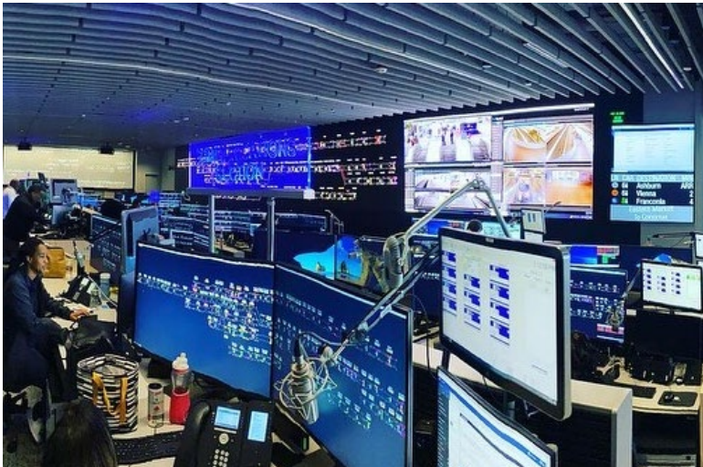
Metro Integrated Command & Communications Center (MICC)
